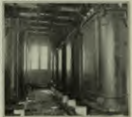
TRANSFORMERS IN TRANSFORMER STATION
